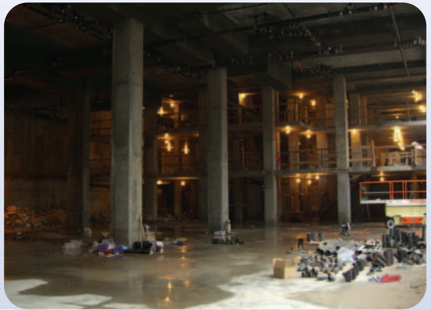
The interior of the StreetSquash Squash Courts, looking into the locker rooms, offices, and classrooms.
